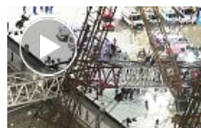
Crane collapses at Mecca's Grand Mosque
